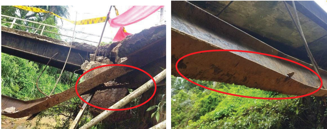
Fig. 6. Visible Corrosion and the area loss due corrosion of the deformed beam
