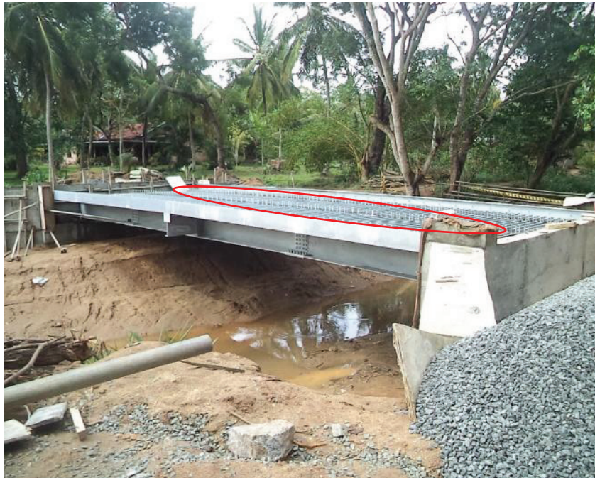
Fig. 12: Bridge deck of having shear studs welded to top flanges of supporting beams
