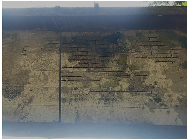
Fig. 7. Exposed reinforcements of the deck slab
