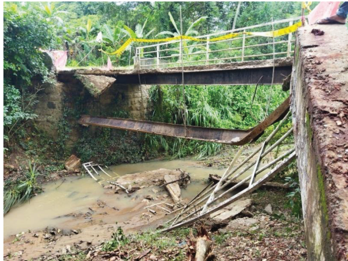
Fig. 5. Extensive later deformation of edge beam
